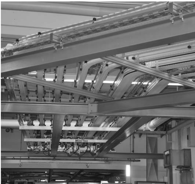
Transportation of coffee doses below hall roof
